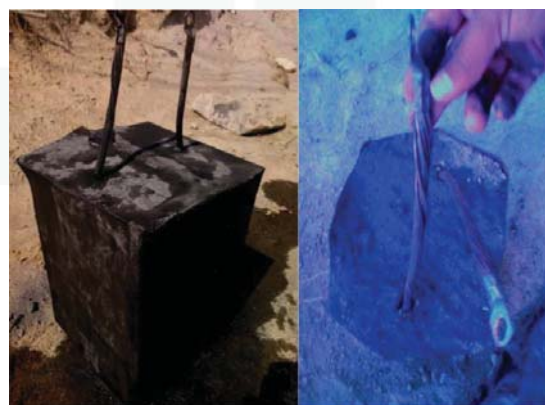
Figure 1: Implementation of portable grounding system
